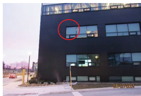
h- Visible thermal bridging through window frames and building envelope studs
