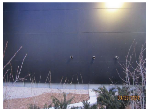
p- Thermal bridging through steel cladding and venting pipes
