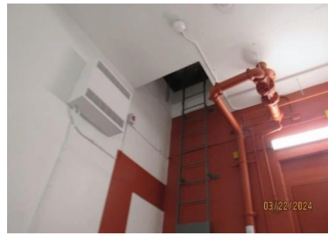
j- Visible thermal bridging through roof hatch
