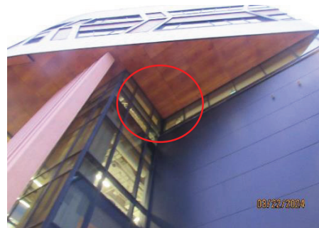
n- Thermal losses through the ceiling due to stack effect
